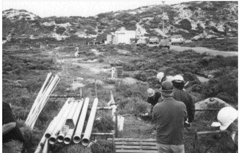
Stainless steel pipe laid out before installation: air sparging well at test site in southern California.
