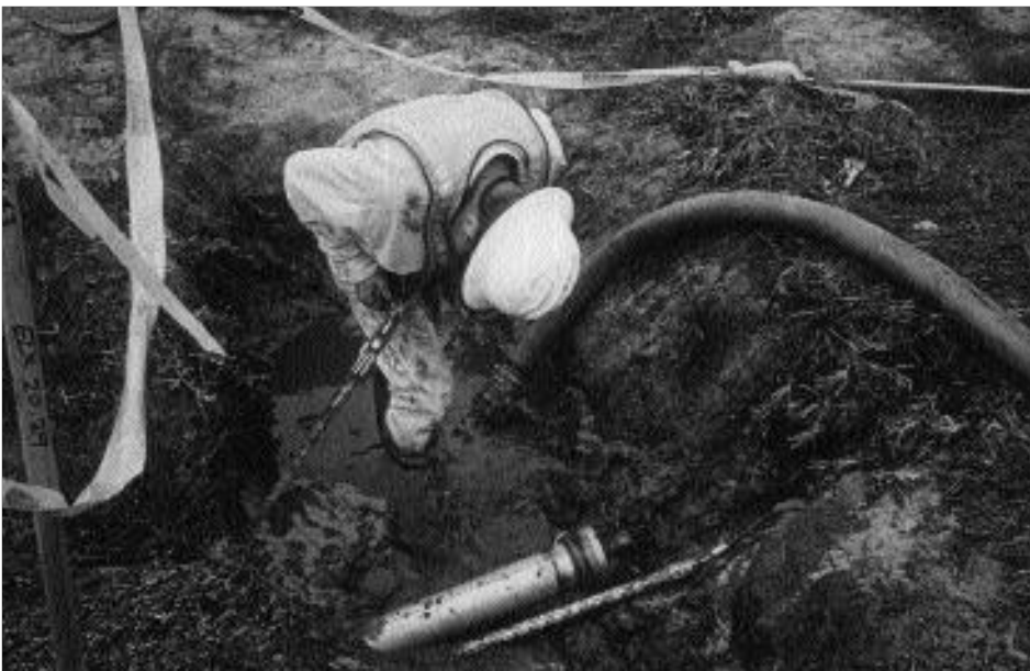
Horizontal well head for air sparging well in southern California.
